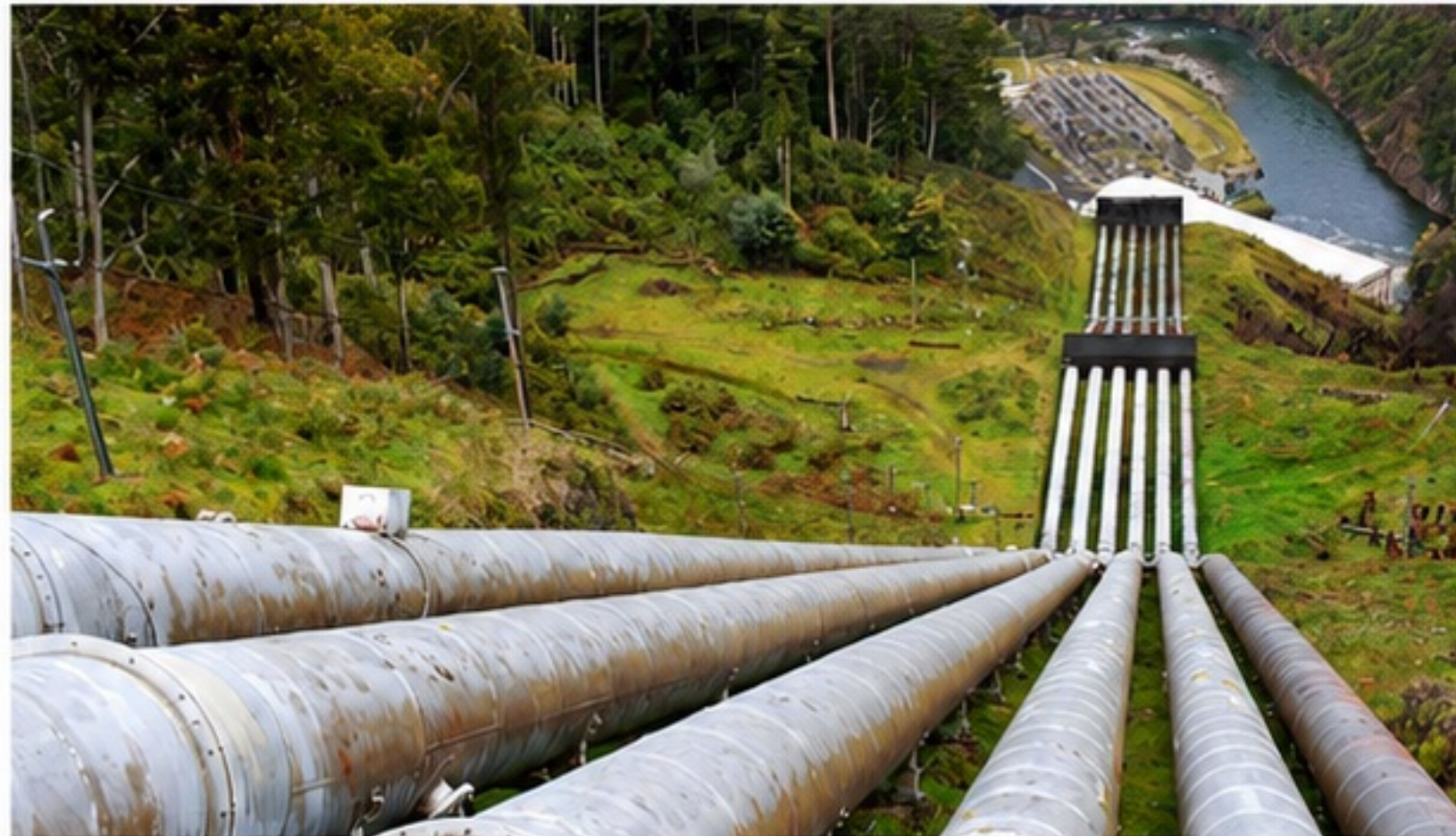
A pumped hydroelectric storage power plant in Tasmania. The plant stores electricity by pumping water uphill when power is abundant. Later, generating electricity downhill through turbines, generating electricity during periods of high demand. GETTY IMAGES
